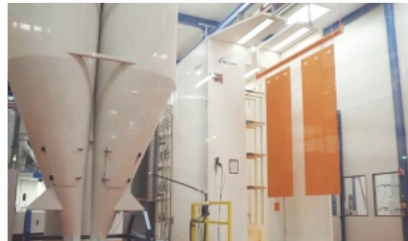
Fully automated state-of-the-art paint plant
